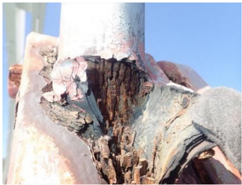
損傷箇所①
